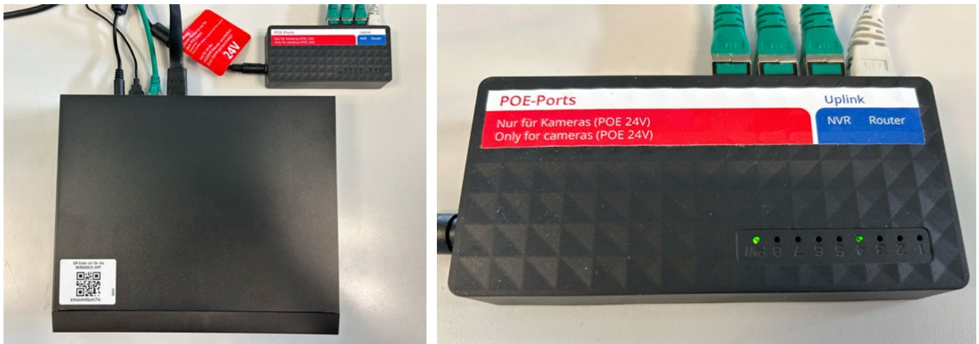
Picture 2-3: NVR + PoE switch setup
