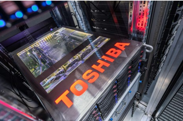
Server and Storage in the Technology Experience Lab (Copyright: © NTT – Global Data Centers)
